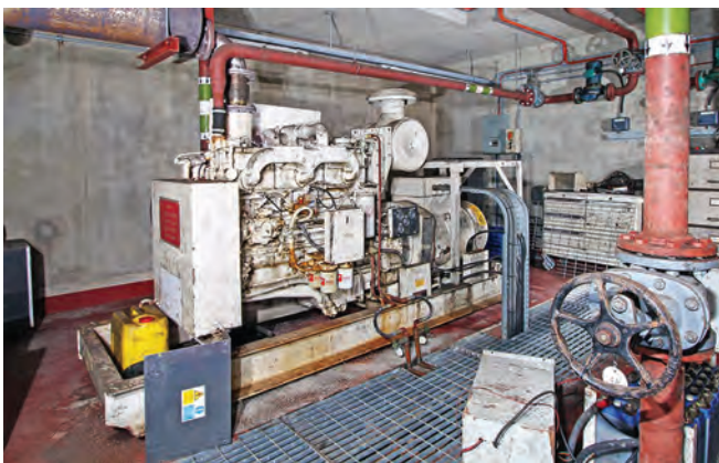
One of the two diesel generators
